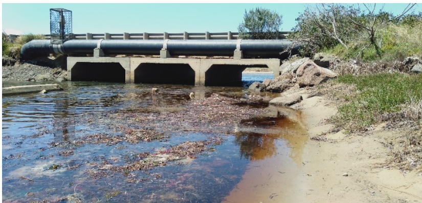
Figure 51: Causeway with four new culverts, Point Impossible Road, Mullet Creek. Source: Surf Coast Shire.
