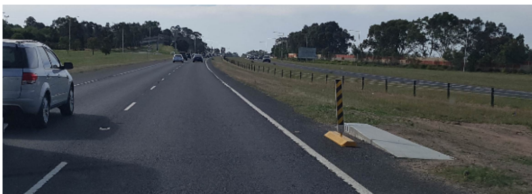
Example of TIRTL installed on the Princes Freeway
