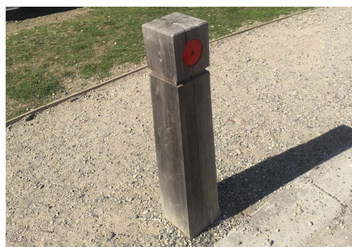
Timber bollards Existing bollards to be retained, separating the car park and pedestrian spaces.
