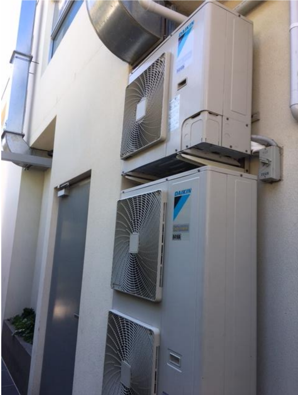
Figure D – Current placement of restaurant air-conditioning condensers which our client wishes to relocate in an effort to resolve any noise nuisance.
