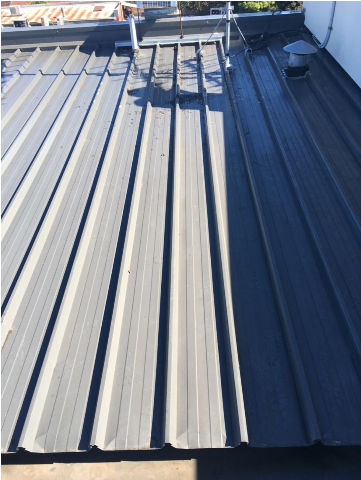
Figure B – Current state of roof as at 29 August 2017 at new duct exit
