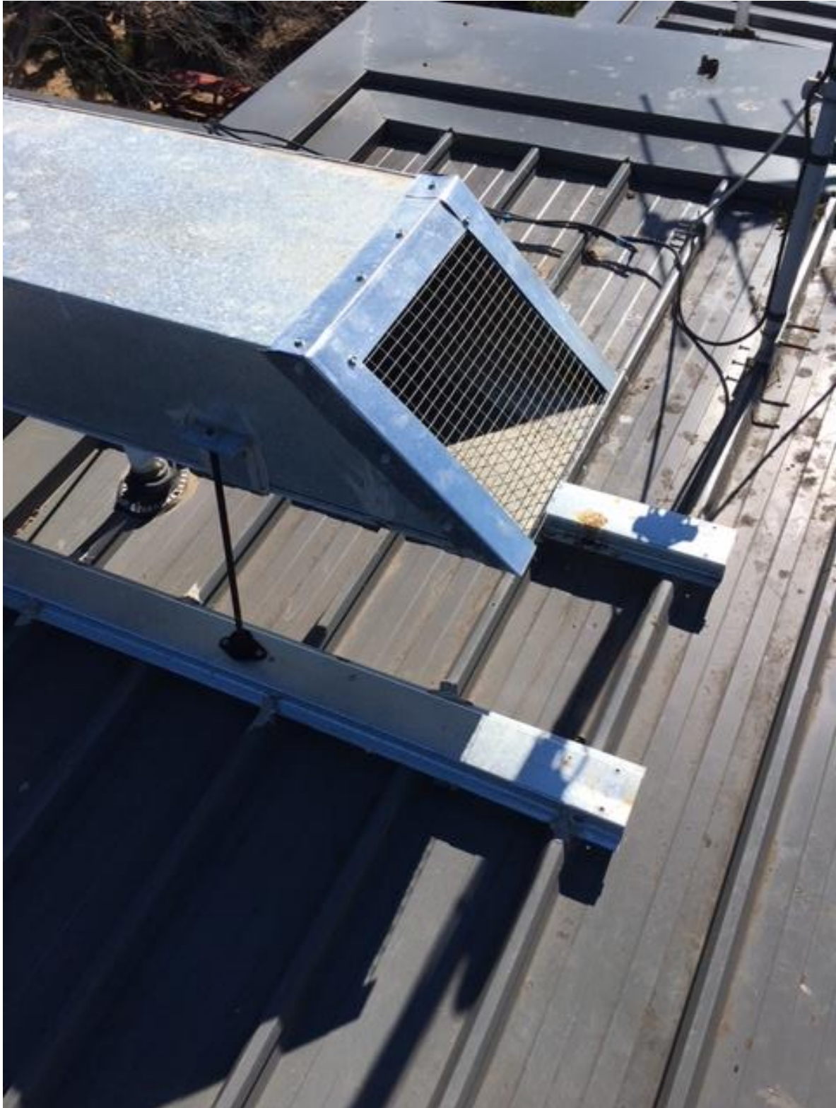
Figure C – Current Duct up-close showing no grease from new system inside or out (nb: bird droppings beside)
