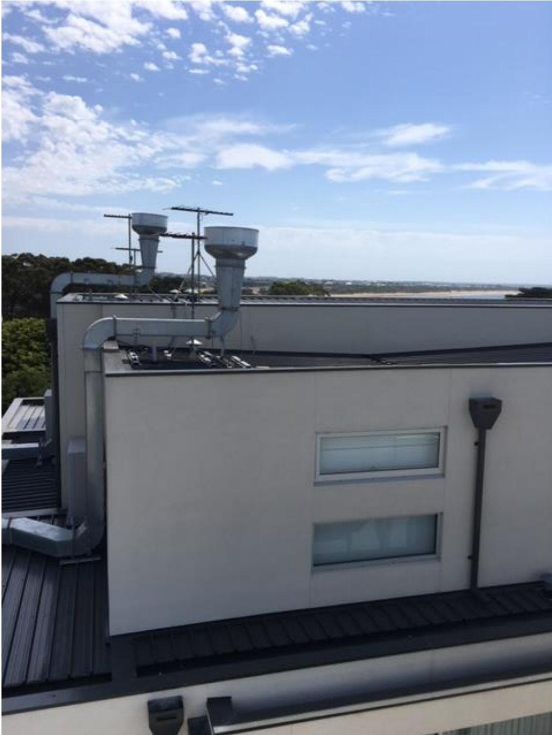
Figure A – Previous exhaust stack discharge with top mounted fan which caused roof grease
