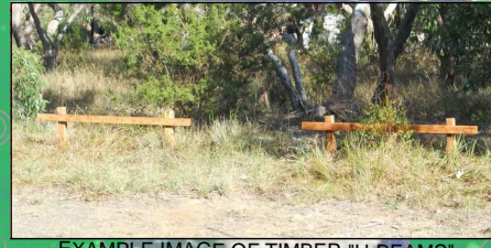
INSTALLATION OF TIMBER "H-BEAMS" (TWO BOLLARDS WITH CROSS BEAM) TO RESTRICT VEHICLES ENTERING ADJACENT VEGETATED AREAS. LAYOUT INDICATIVE ONLY.
