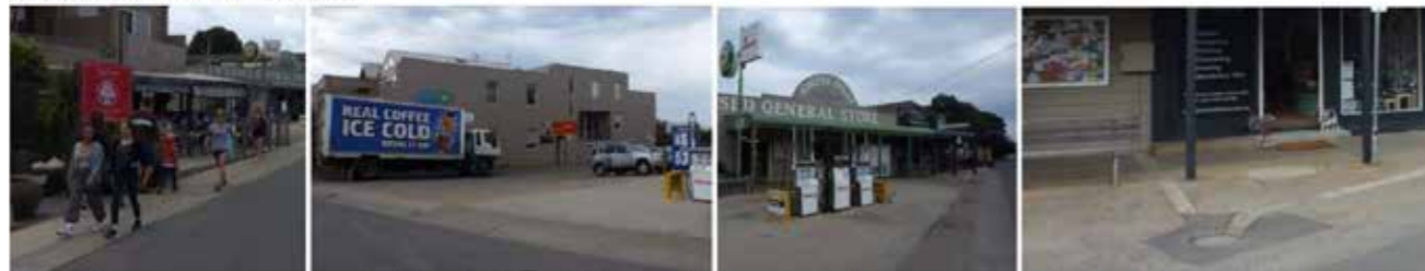
Narrow footpath Conflict point for pedestrians and vehicles at petrol bowers and car park Uneven concrete surfaces
